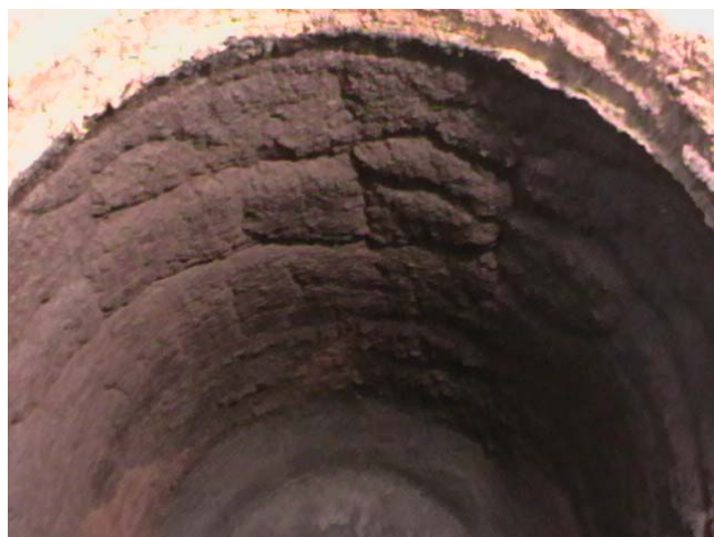
Fig. 2: Photo of a severely damaged furnace wall from a 25 t crucible induction furnace
